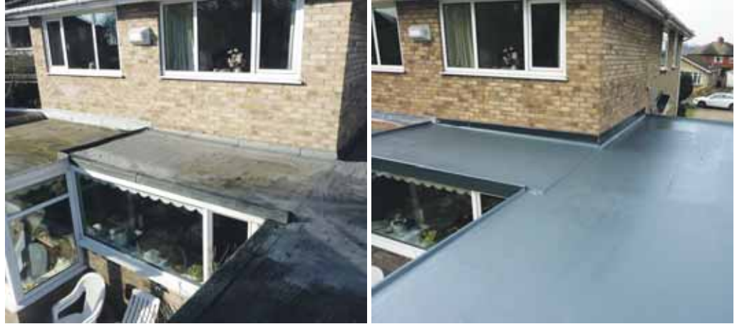
Roof in its original leaking state
